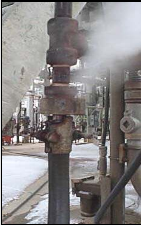
Steam leak at the coupling /spud connection
