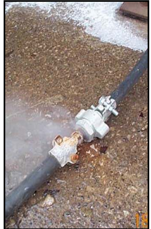
Steam leak at the coupling / clamp
