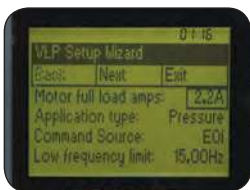
STEP 1: Input Motor's Electrical Specifications
