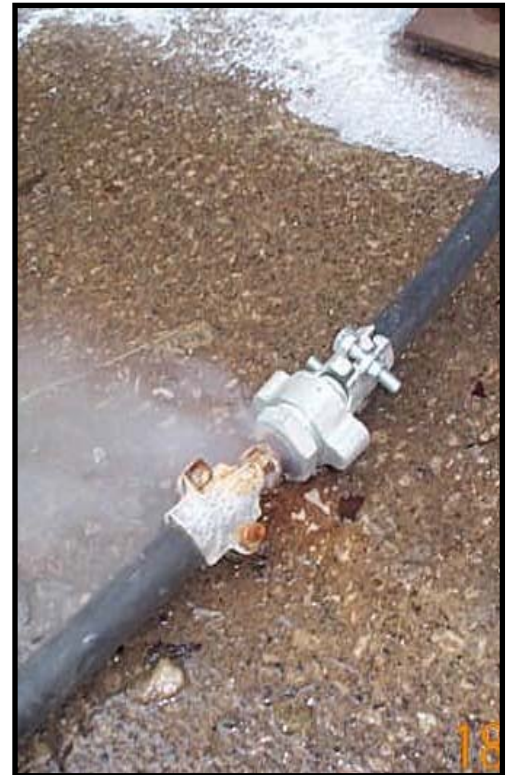
Steam leak at the coupling / clamp
