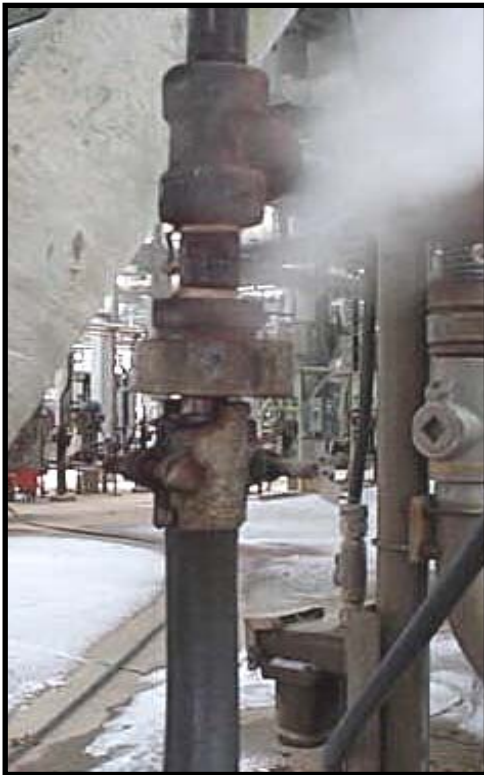
Steam leak at the coupling /spud connection
